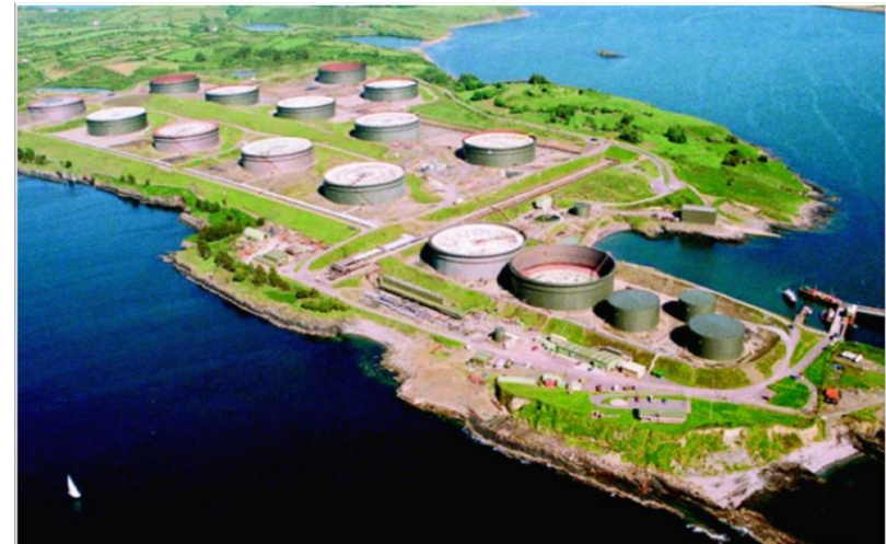
Bantry Bay Oil Storage Facility
